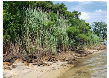
BIL funding will be used to restore eroding shorelines like this one at Assateague State Park.
