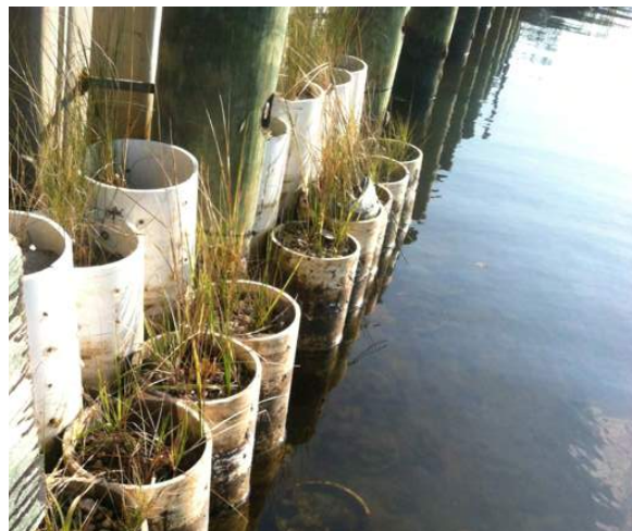
The completed installation of a green bulkhead in Ocean City. Grasses are planted in the top of these PVC pipes to provide additional habitat for fish and other aquatic species. Photo by Roman Jesien.
