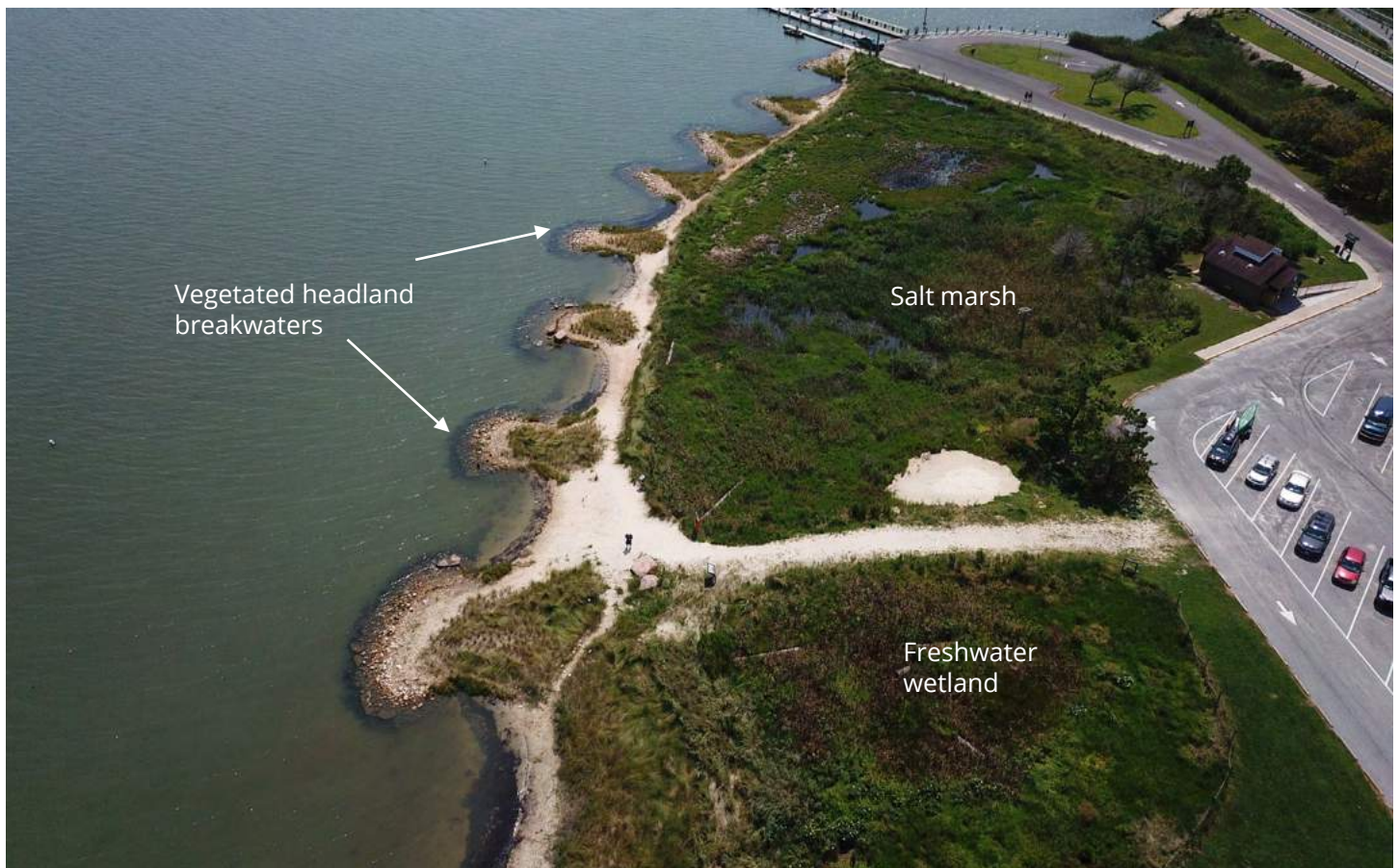
The living shoreline project near the Assateague State Park boat ramp. Eroding shoreline was enhanced with headlands and beaches that dissipate wave energy and a freshwater wetland that intercepts storm water. White sand in the center is a diamondback terrapin sanctuary that also provides space for nesting. Photo by Roman Jesien.
