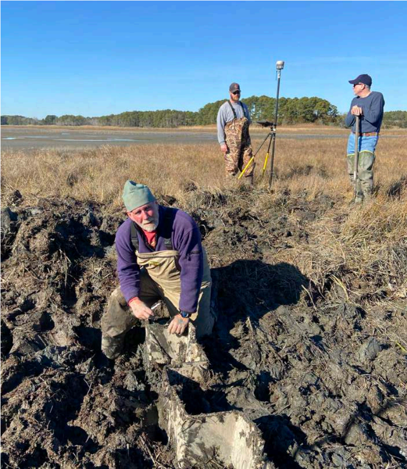
U.S. FWS, UMCES, and MCBP staff modify earthen and sheet pile plugs from mosquito ditches constructed in the early 1900's. Proper hydrology is critical to maintaining healthy and robust marsh ecosystems.
