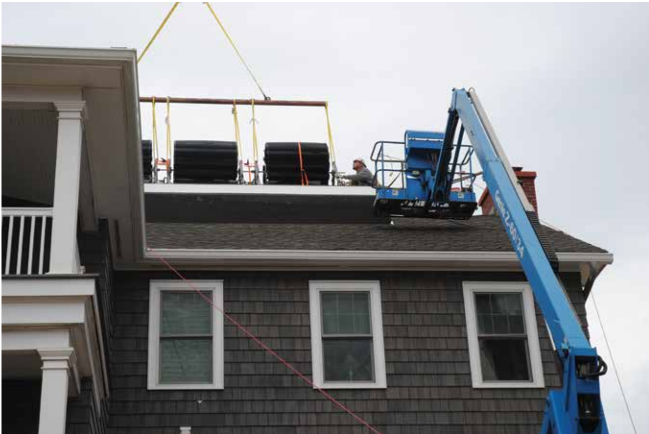
Workers install the first residential wind turbine in Ocean City on the Boardwalk at 14th Street. The new system should produce around 61,000 kilowatts of electricity each year—enough to power the condo for the summer. Photo courtesy of Ocean City Today.
